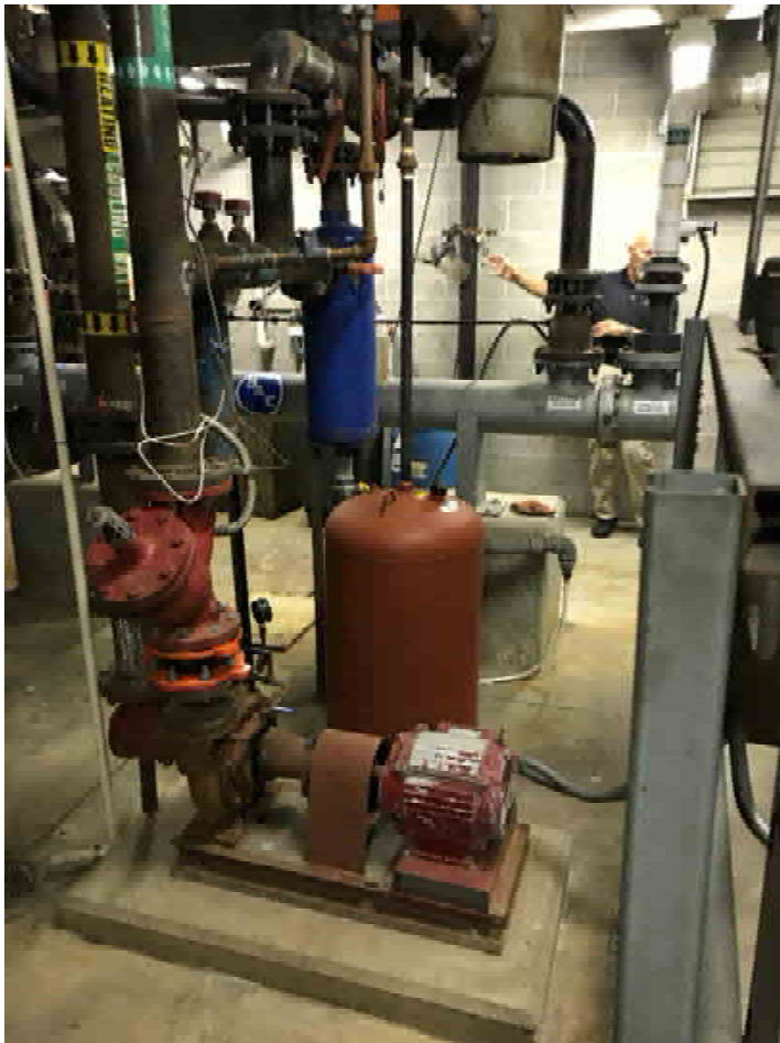
Circulation Pump for Water-Source Heat Pumps
