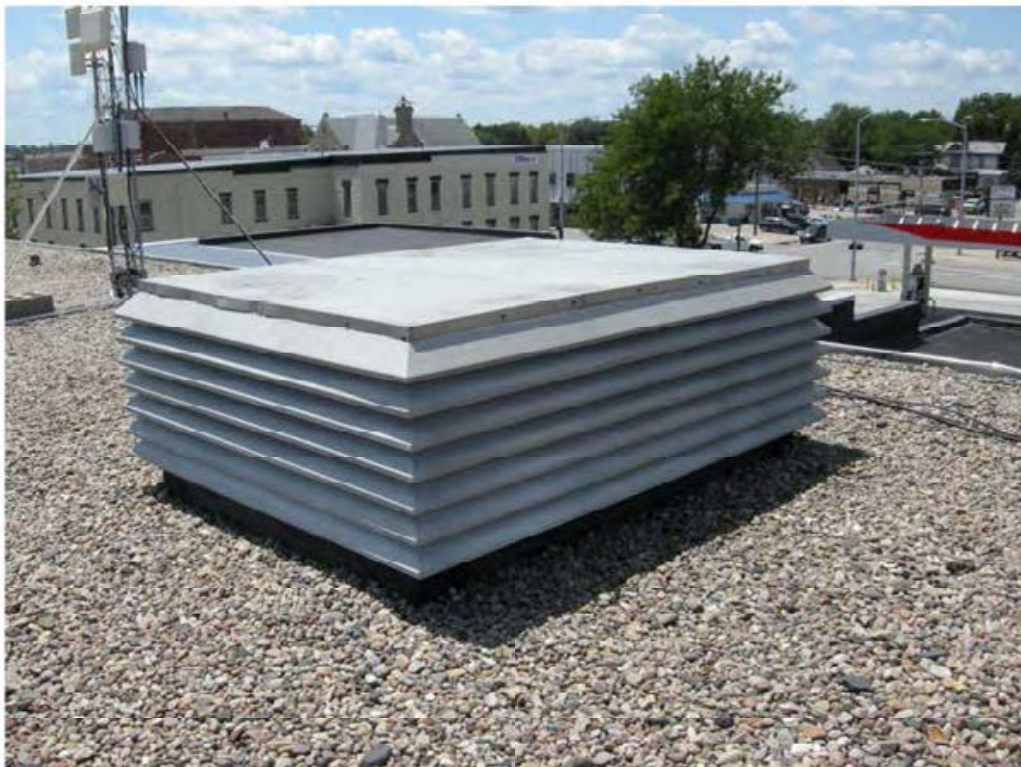
Roof mounted outside air intake for the air handler.
