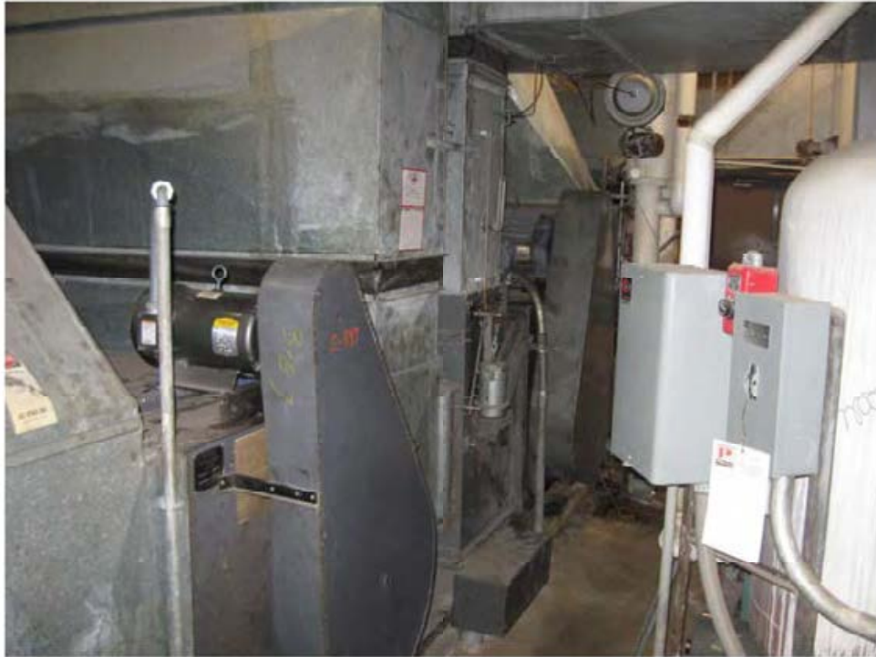
Original "dual-duct" air handler located in the basement.
