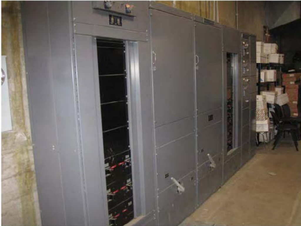
Main switchgear in basement
