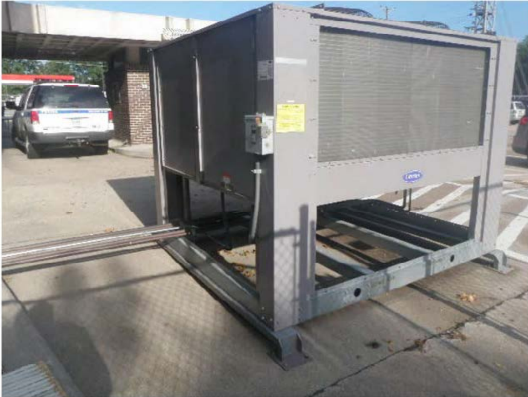
Existing air-cooled condensing unit located outside the northeast corner of the building.
