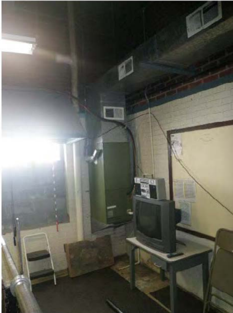
A self contained package unit, manufactured by Rheem, provides 1,200 cfm of heating and cooling air to the exercise room.
