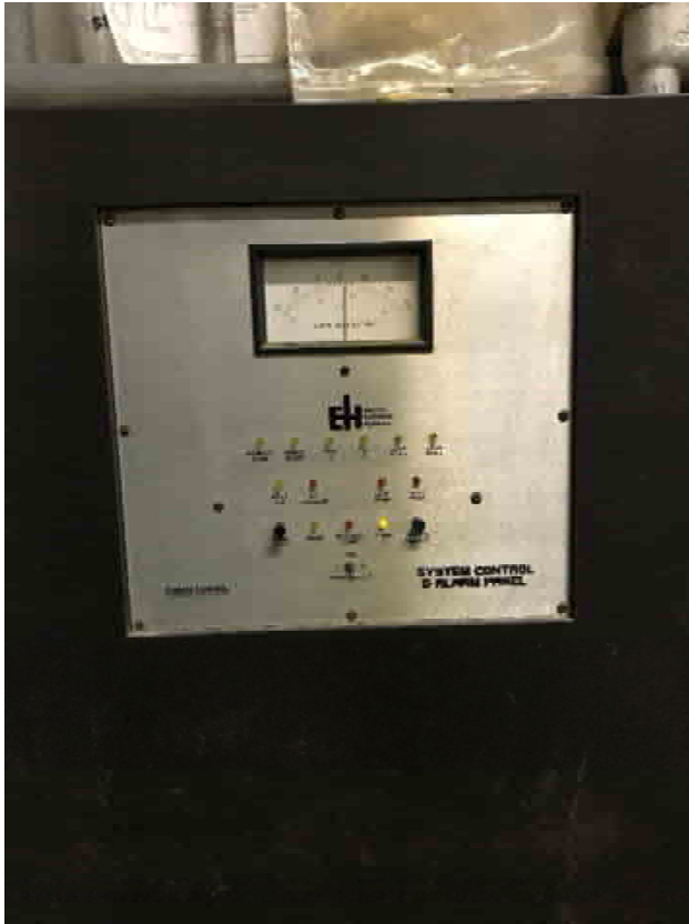
Controller originally for the now-removed Fluid Cooler.
