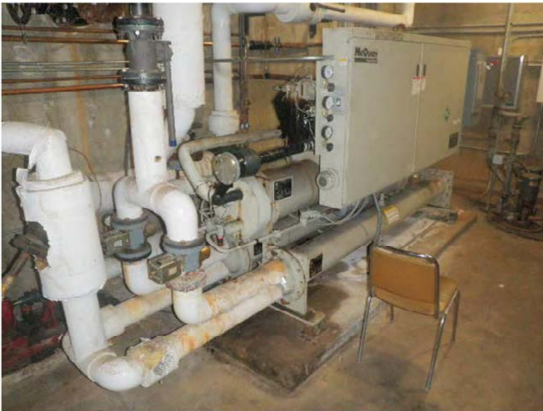
Existing chiller located in basement
