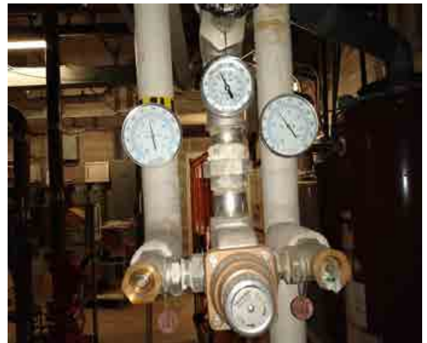
Figure 3: Thermostatic mixing valve regulating domestic hot water temperature. Thermometer measuring cold water temperature reads 108 F, indicating the integral check is not seating properly.
