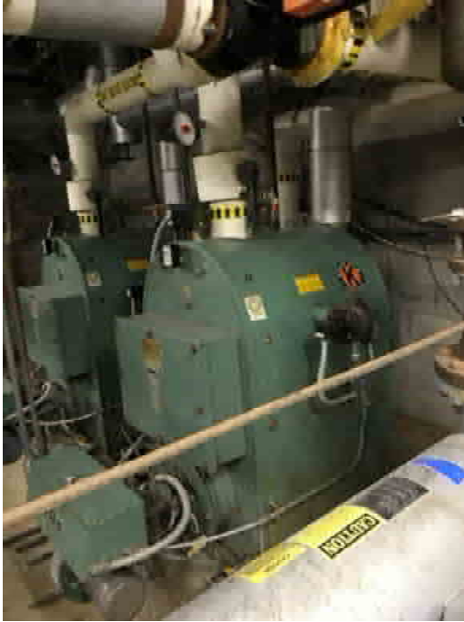
Hot Water Boilers for Heating
