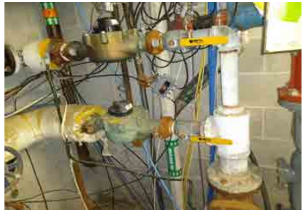
Figure 2: Existing stacked water meters with fiber optic and other cabling strewn over the years contributes to cobbled appearance.
