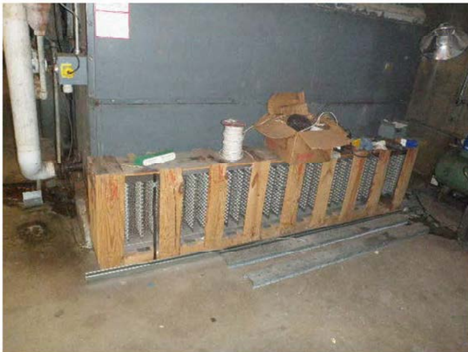
Replacement 150 kW electric heating coil, still in crate.
