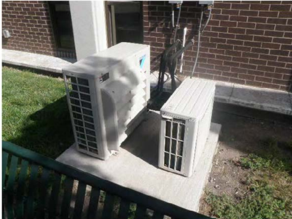
In spaces with heavy electronic equipment, such as Dispatch, separate ductless split system air conditioners have been added to provide additional cooling capacity.
