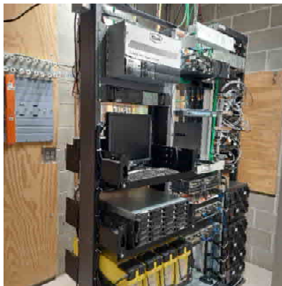
Figure 74: DMP Fire Alarm serviced by SEI
