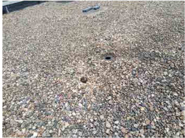
Figure 1: Primary roof drain with dome missing and field-fabricated wire mesh used to protect the secondary roof drain from debris.
