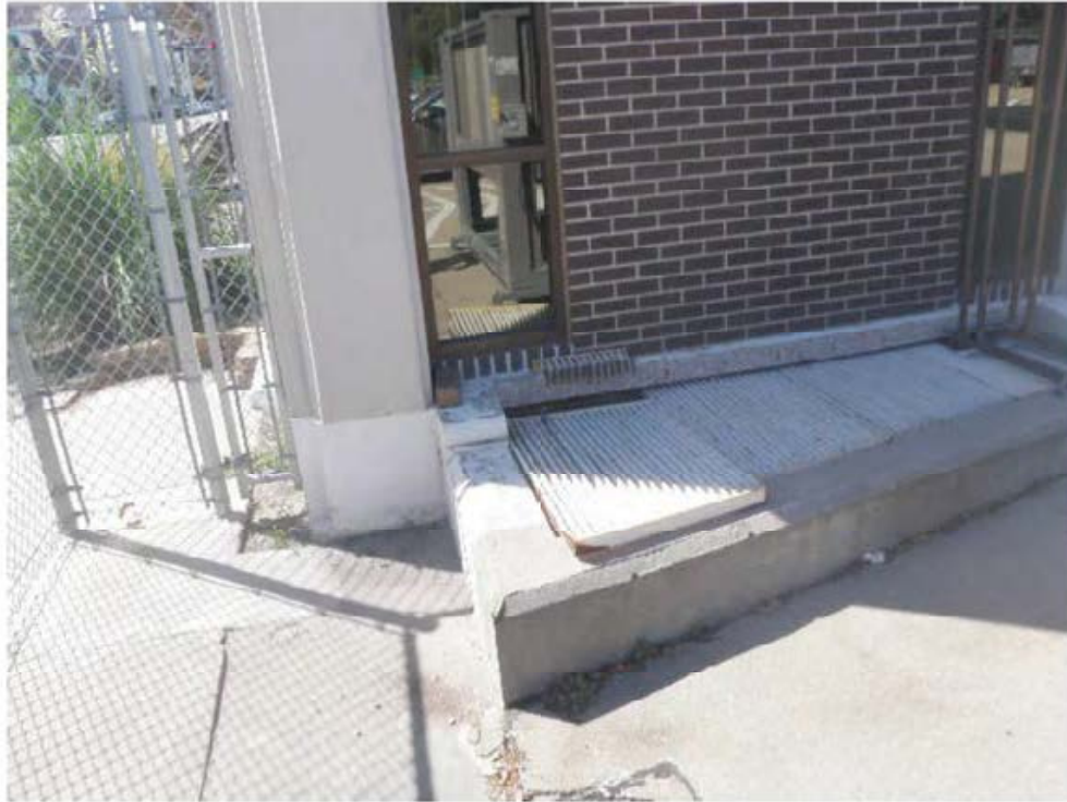
Area way for relieving air from the basement air handler. (This previously provided equipment access to the basement, but is now no longer usable for basement access.)
