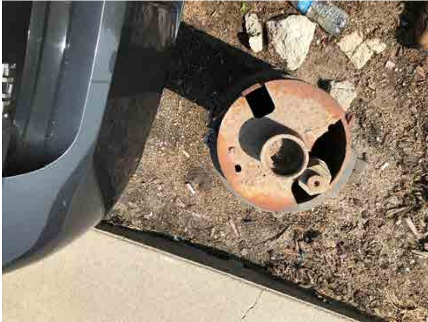
Re-injection Well (Unused)
