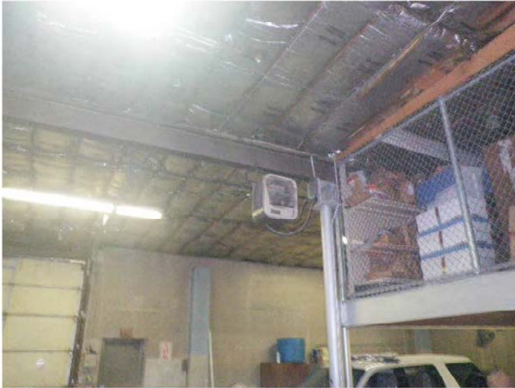
An electric hanging unit heater provides minimal heating to the space over the winter.
