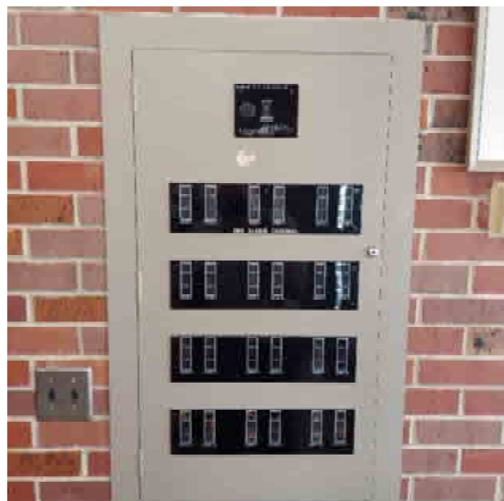
Fire Alarm Panel
