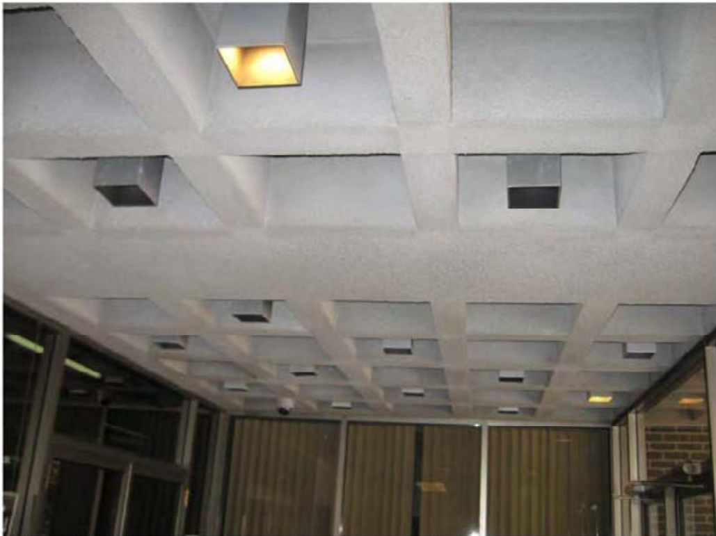
Original light fixtures in Vestibule – note only two are lit (exterior canopy similar)
