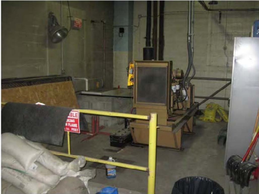
Emergency generator located in garage
