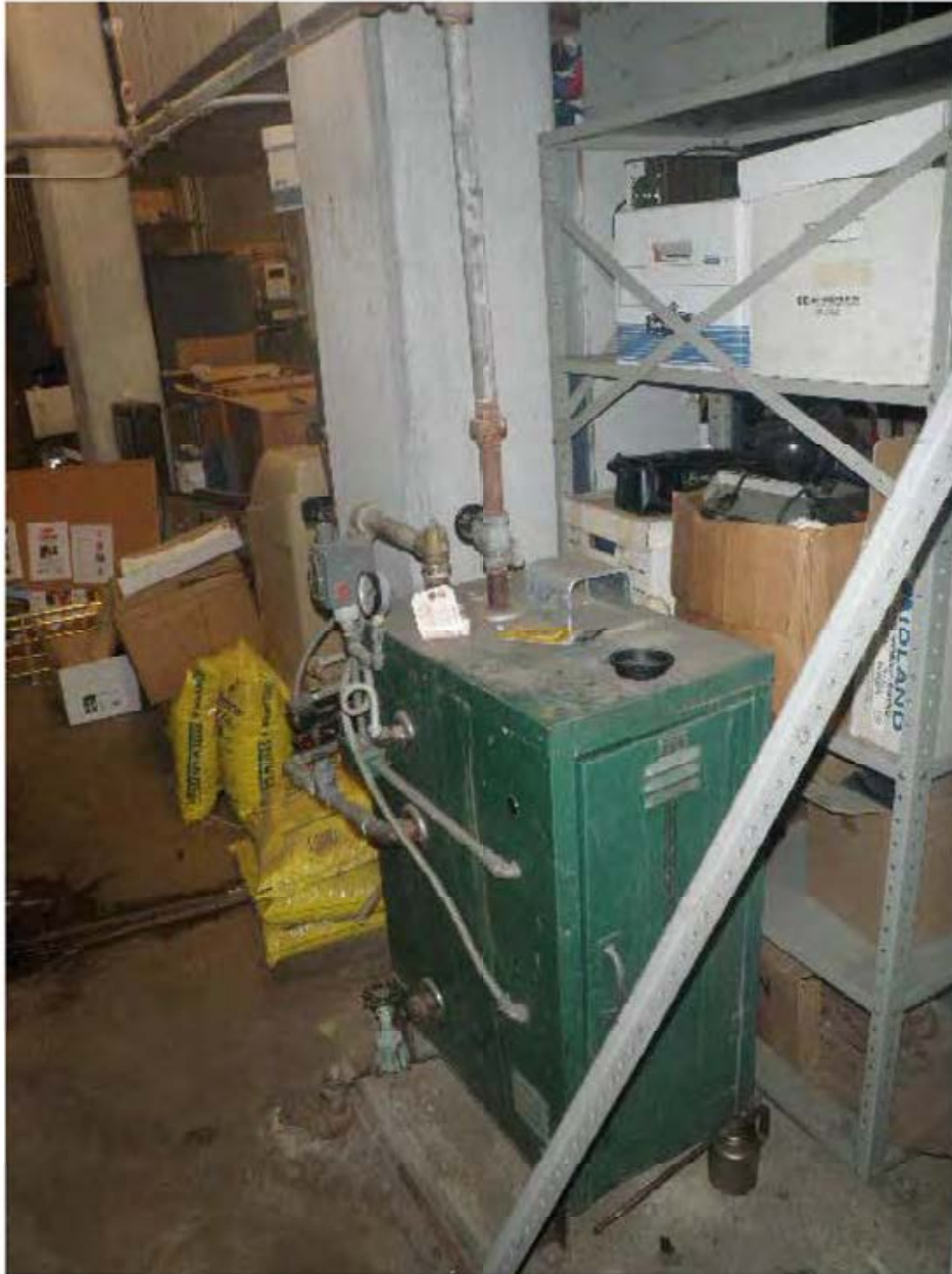
A 48kW electric resistance boiler served by a water softener provides steam to the air handler for building humidification in winter.
