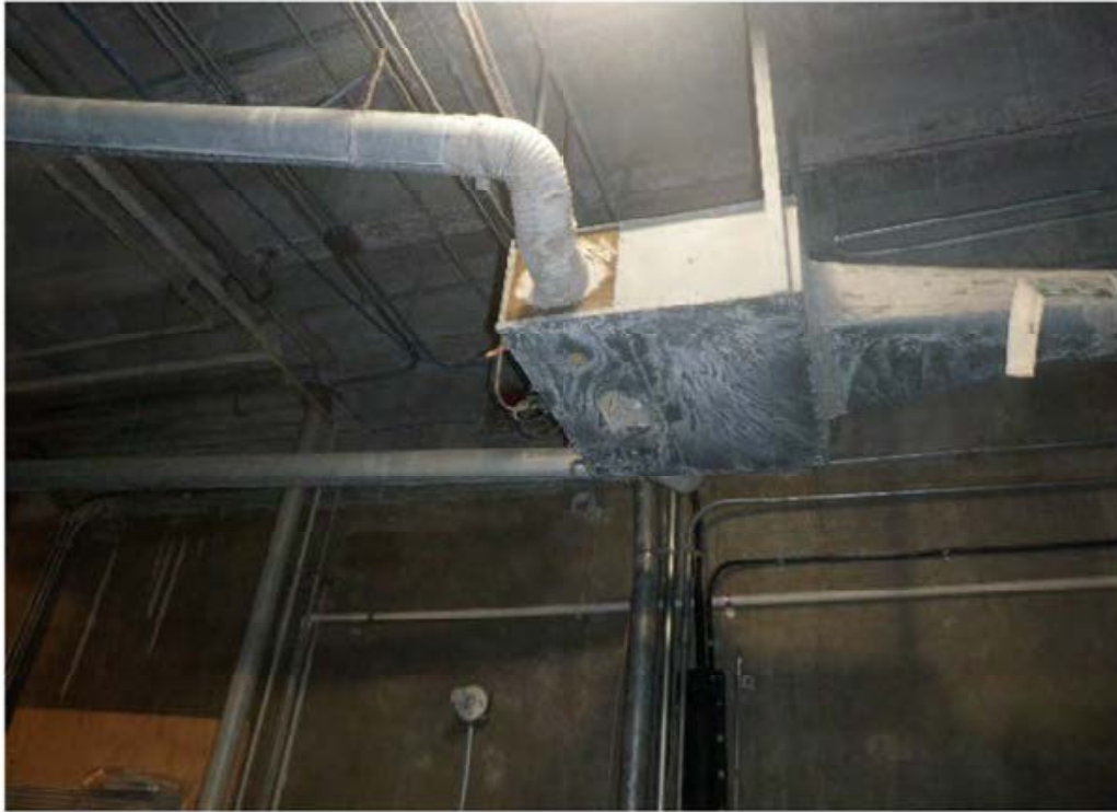
Example of a “dual-duct” mixing box with both hot and cold duct connections. White streaking on box is from outside water leaking into the building, entering the ductwork, then the basement.
